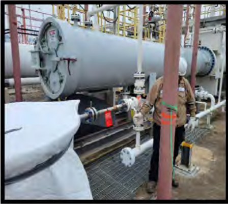
Leak Detection System Test BH CO Pipeline
