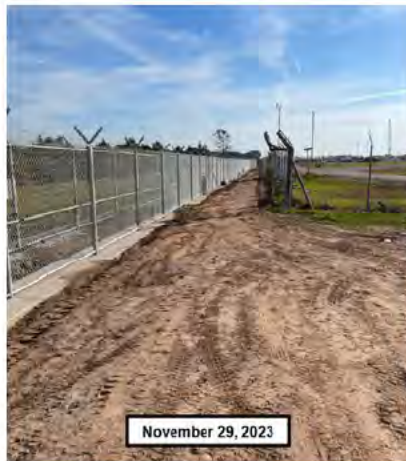
November 29, 2023 BH-LE-1735 – Fence fabric installed along the West end of the North perimeter (CWA-80)
