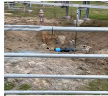
Fire Water Failure
