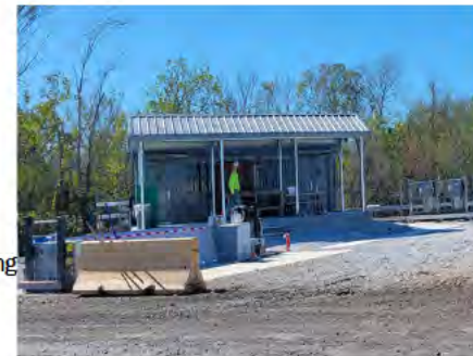
BC-LE-1723B, New Contractor Screening Portal and Mobile Wedge Gate Barrier at the Brine Road gate
