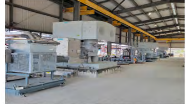
BC-LE-1759, The Three New 3500 HP Raw Water Injection Pumps
