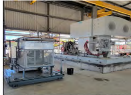
BC-LE-1759, New Raw Water Injection Pump, Motor, and Oiler Skid
