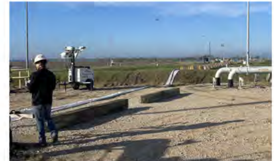
Cavern 112 - Cavern 109 temporary piping
