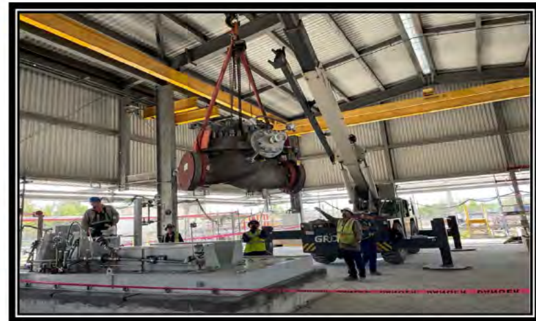
BC-LE-1759, LE2 Consolidated Work Package Observation for the weeks of October 23, 2023 Raw Water Pump Critical Lifts
