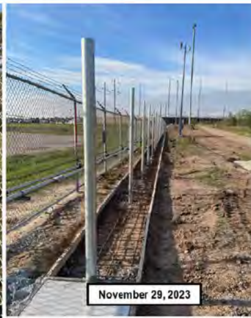
November 29, 2023 BH-LE-1735 – New fence posts and apron forms along East perimeter CWA-81
