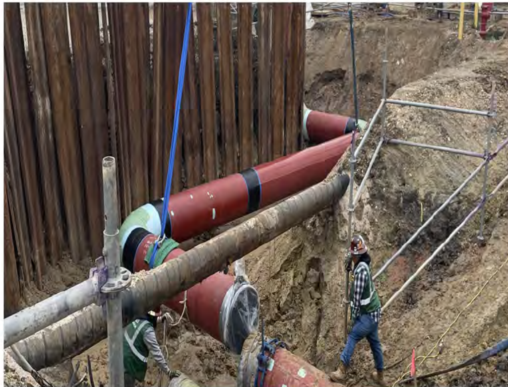
LE2 Piping – System 32
