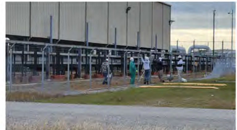
Security Fence Deflection
